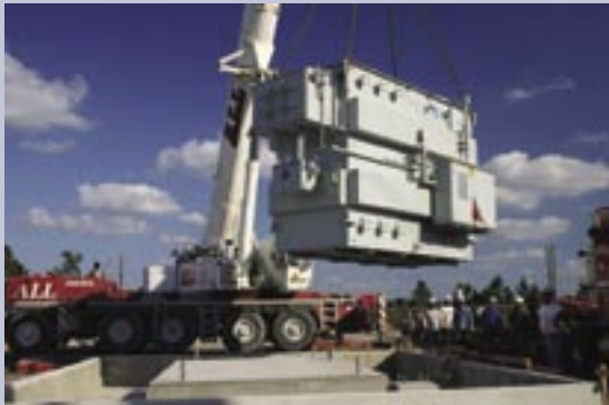
New substations, like this one in Manatee County, are needed to provide reliable power for existing members — and new ones moving into the area.
